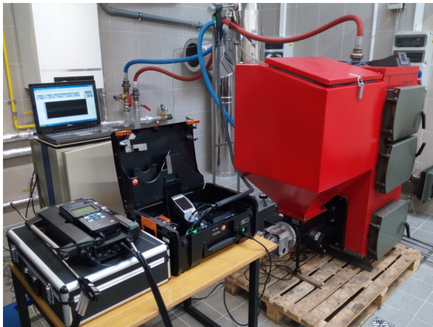
Fig. 2. View of the heating boiler with the test stand
